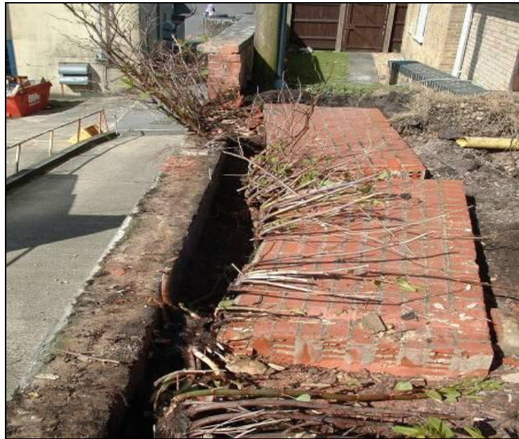
Figure 2.9: A wall undermined by Fallopia japonica (Source: Elcot Environmental).
