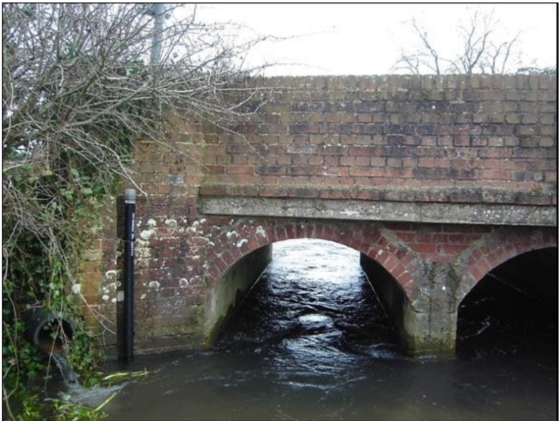
Figure 3.10 - The location of the stilling well that was installed on the Bere Stream at Snatford Bridge in February 2009. Photograph taken by G. Davies.
