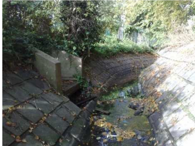
Figure 4.22 View of Mayes Brook at Stretch 1 [MB_001WC] at the time of survey, showing full reinforcement of banks and bed during low or dry weather flow conditions
