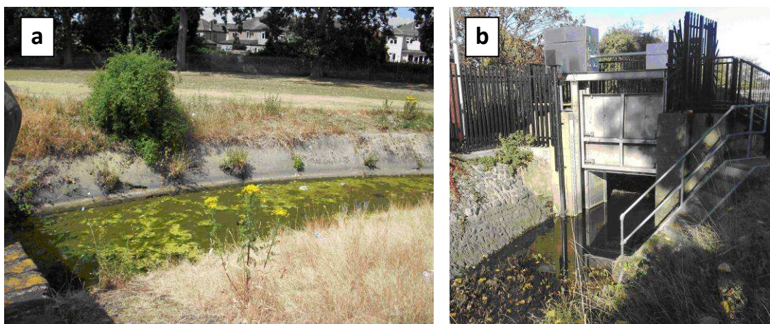
Figure 6.20 Two views of the flood management system at Mayesbrook Park: showing (a) the overflow channel between Mayesbrook and the lakes and (b) the flood sluice gate.
